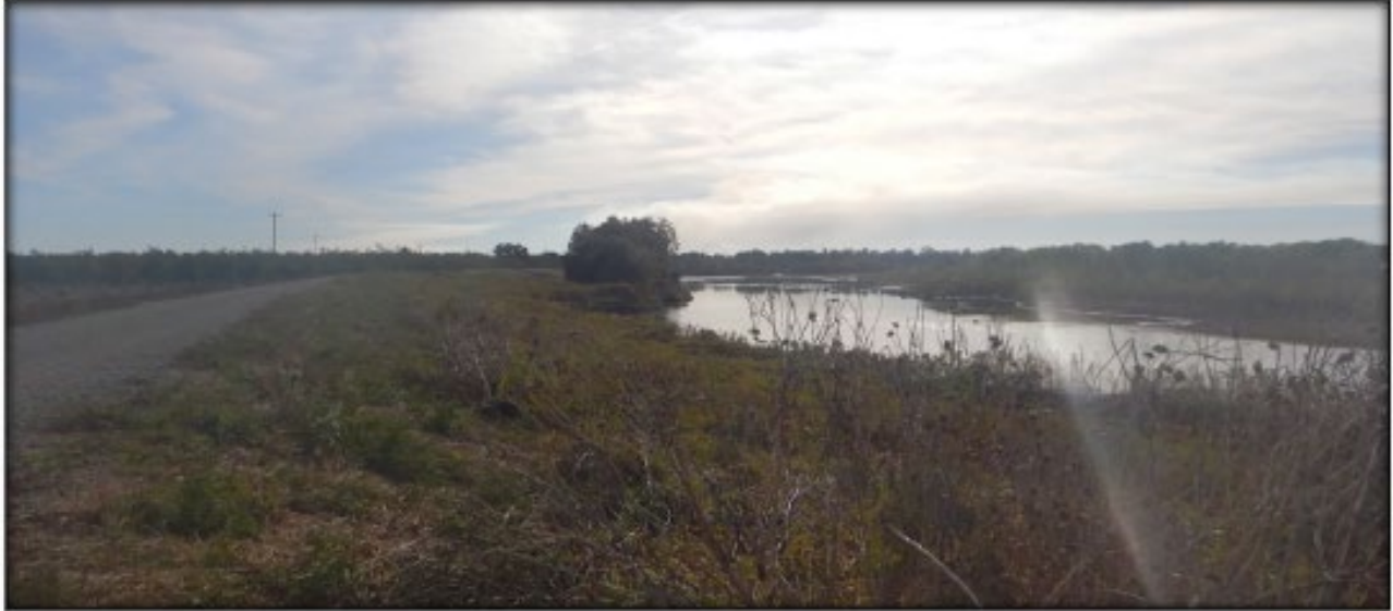
Figure 5 Bank Erosion into the Levee Prism along the Left Bank of the Sacramento River at RM 172.0
