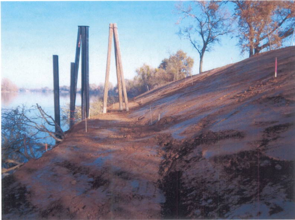
Photograph 1: Lauppe South River Pump site prior to completion of USACE bank stabilization (River Mile 77.3).
