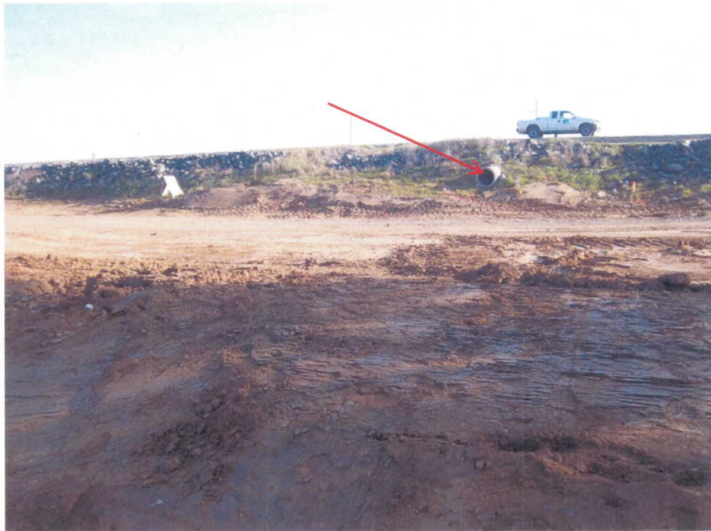
Photograph 4: Looking east toward Garden Highway from Lauppe South River Pump. Arrow points to existing discharge pipe through levee, which is the connection point for the proposed modifications to the Lauppe South River Pump.
