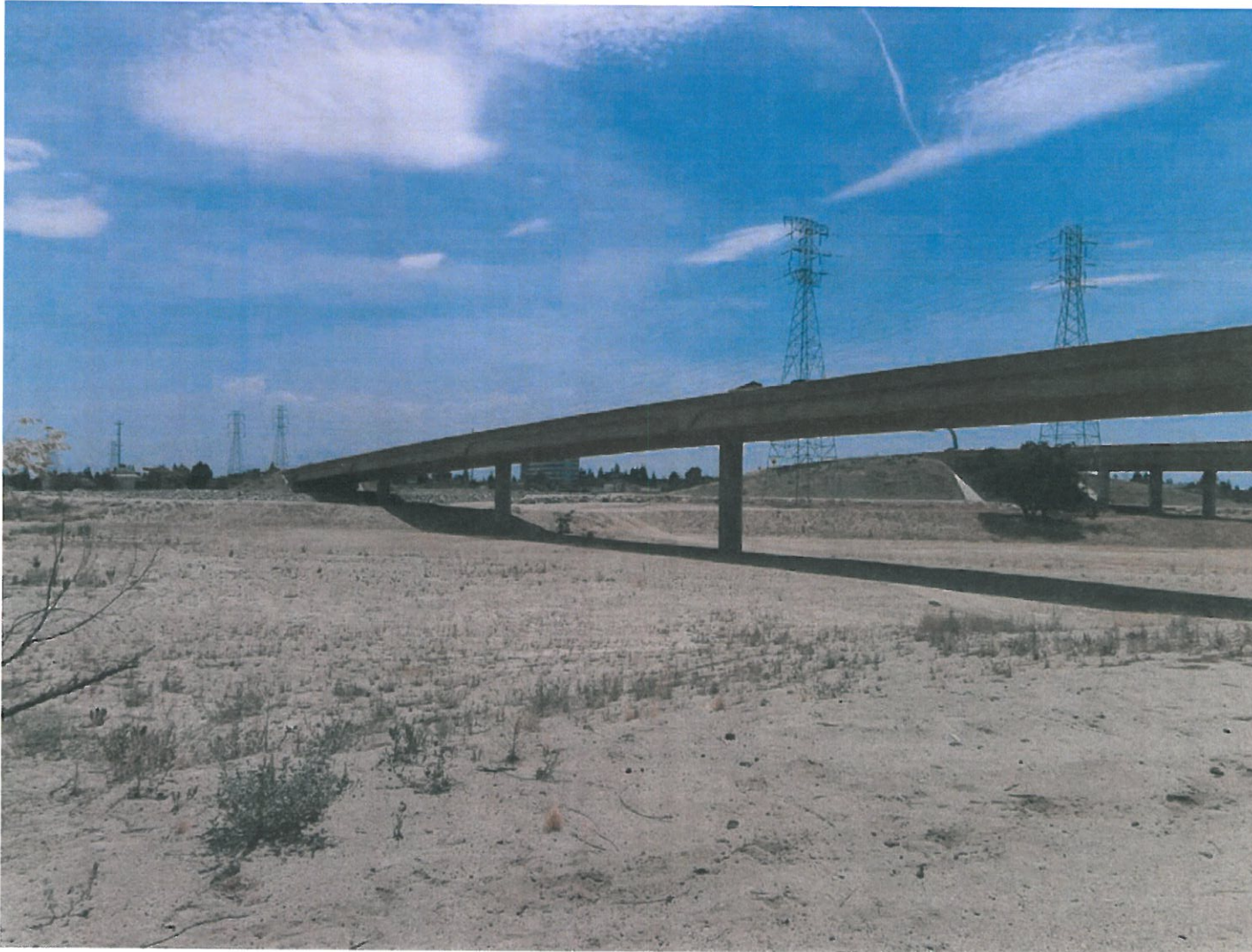
Photo #2 Facing southwest toward Kern River, Westside Parkway, and Truxtun Avenue (June 30, 2015)
