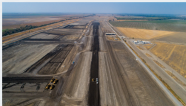
Lower Elkhorn Basin Levee Setback Project under construction in 2021. Photo provided by California Department of Water Resources.
