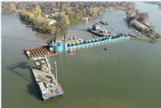
Construction of the Smith Canal Gate Project in 2020. Photo provided by Kjeldsen Sinnock Neudeck.
