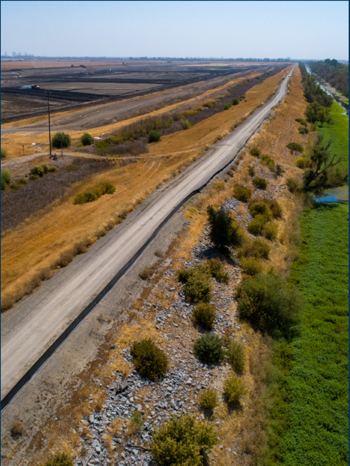
The California Department of Water Resources is constructing setback levees along the Sacramento and Yolo bypasses as part of the Lower Elkhorn Basin Levee Setback project. Photo taken August 31, 2021.
