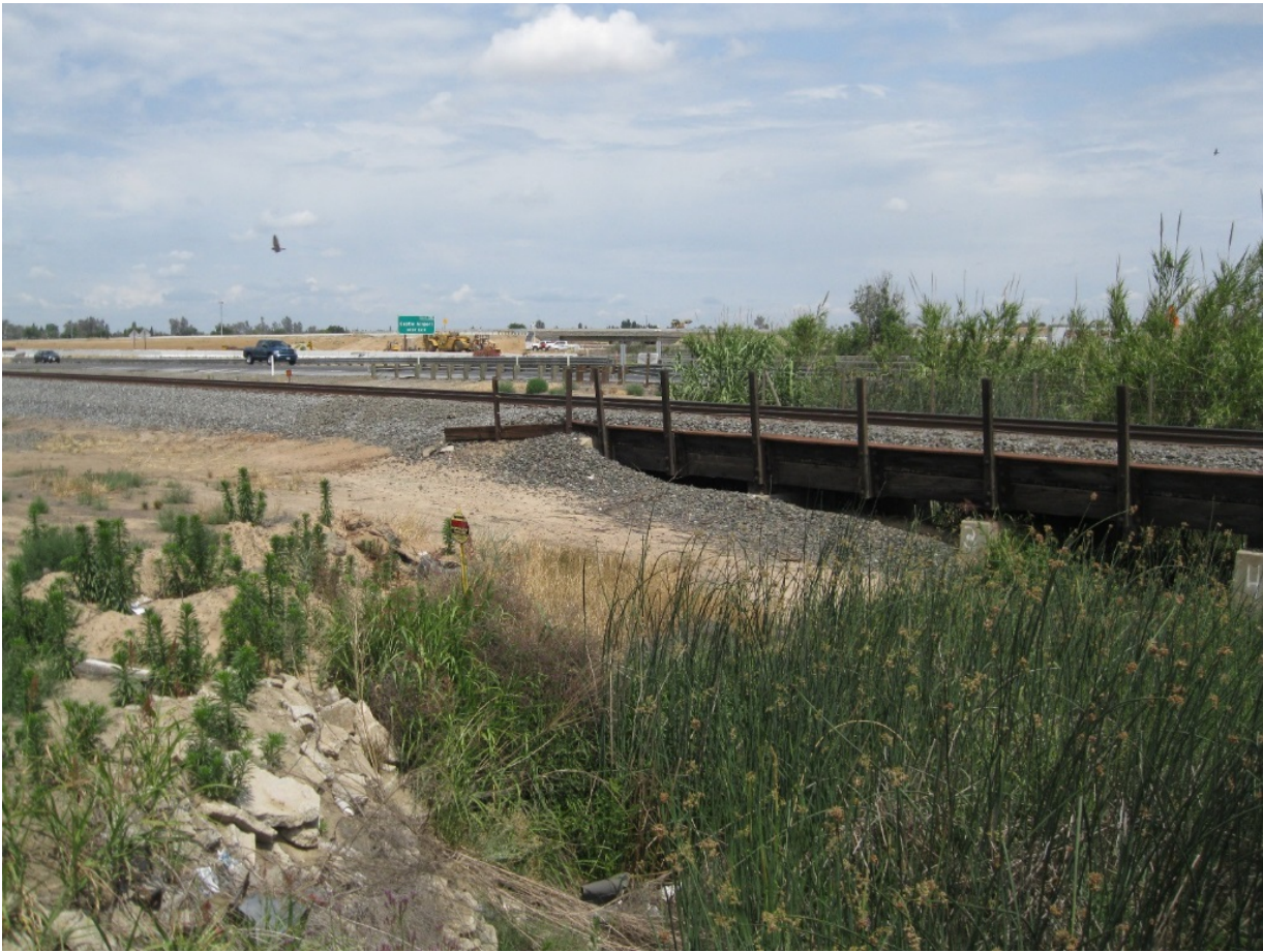
Photograph 1. View of the western ROW and bridge from North Southern Pacific Avenue looking northwest.
