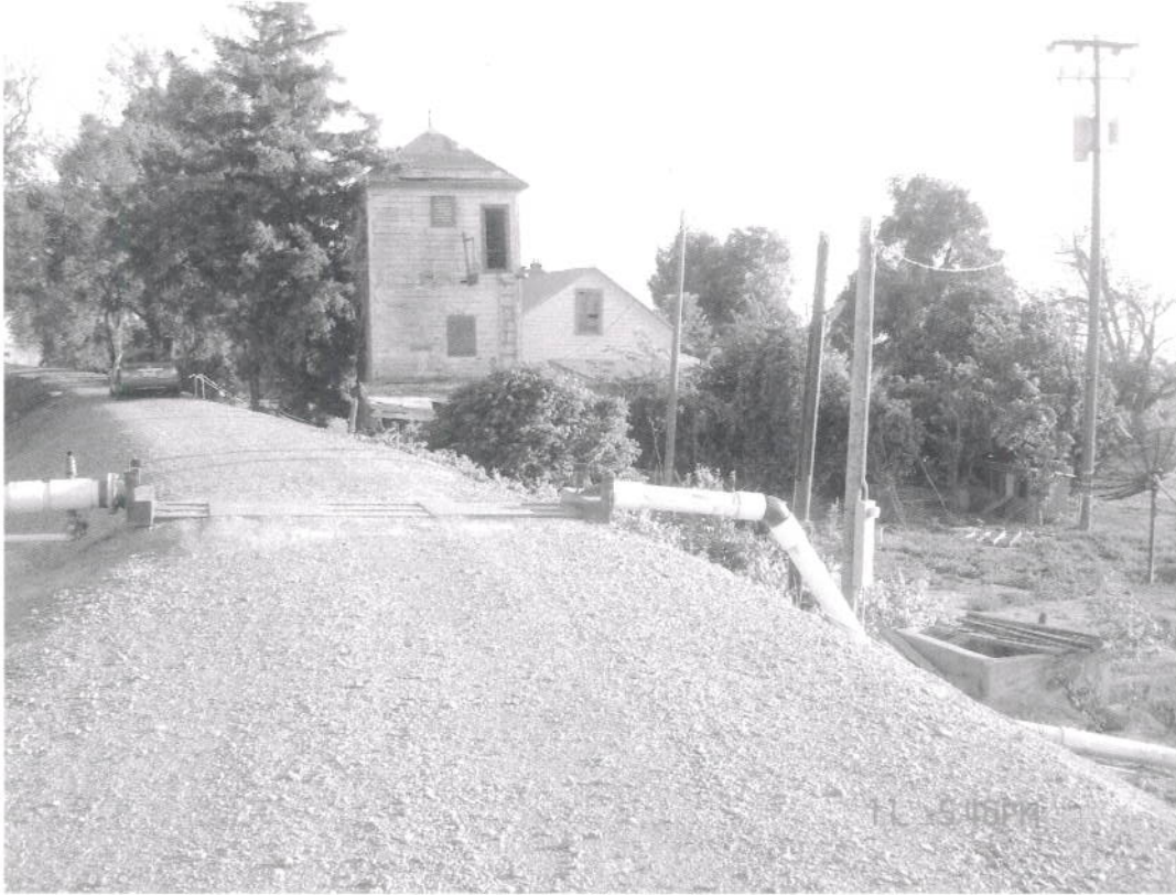
Downstream view of temporary pipe configuration
