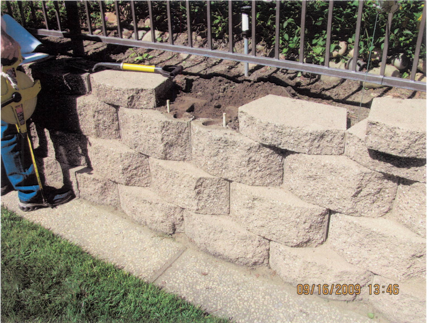
Retaining wall & wrought iron fence along the landside levee toe on Mr. Robles' property
