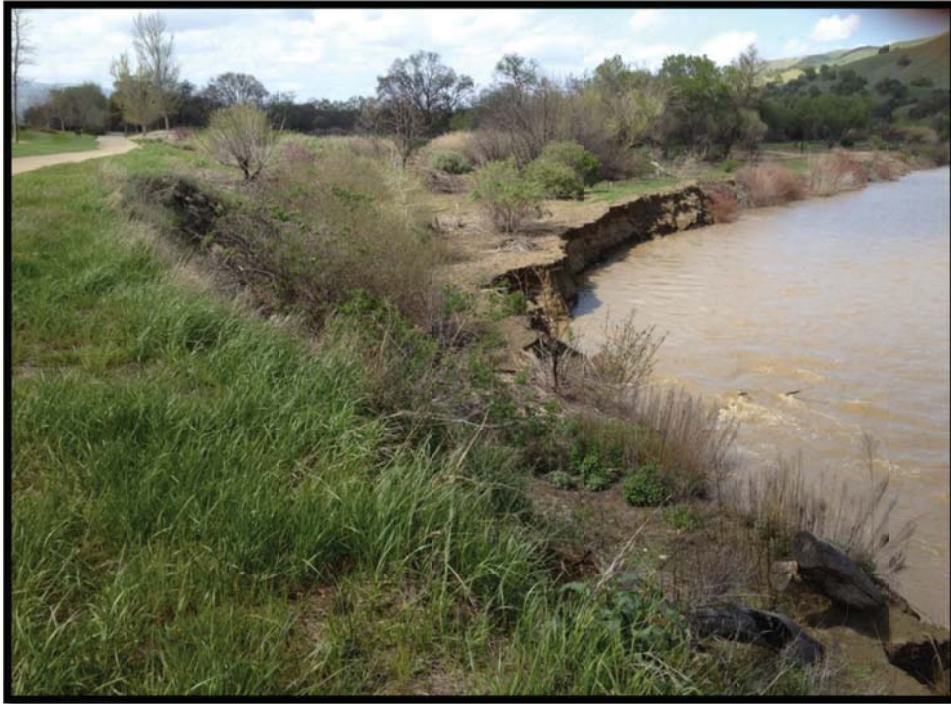
Photo 1: Upstream view of eroding creek bend at project site. The Yocha Dehe Golf Club and cart road border the site to the west. Photo taken during period of high flow March 28, 2012.
