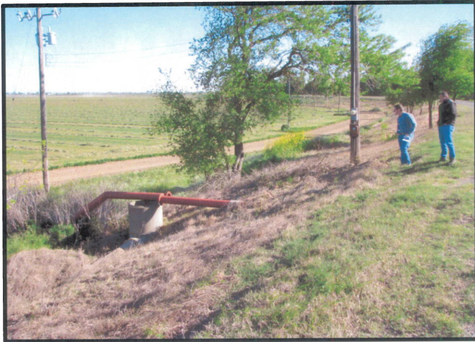
Facing northeast, view of landside slope and encroachment.
