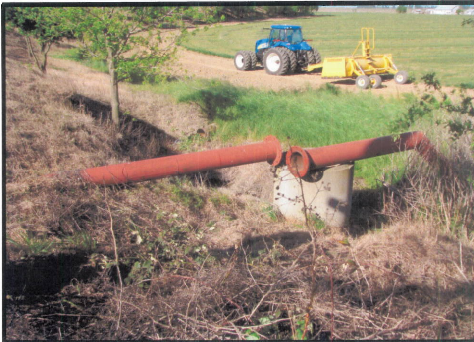
Landside view of encroachment disconnected for maintenance.
