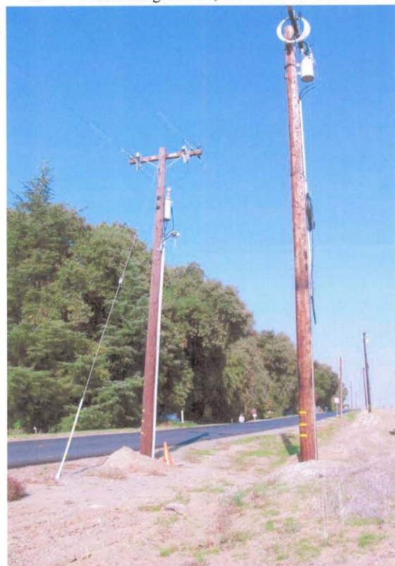
8. Encroaching Pole 97, shown next to Pole 97.
