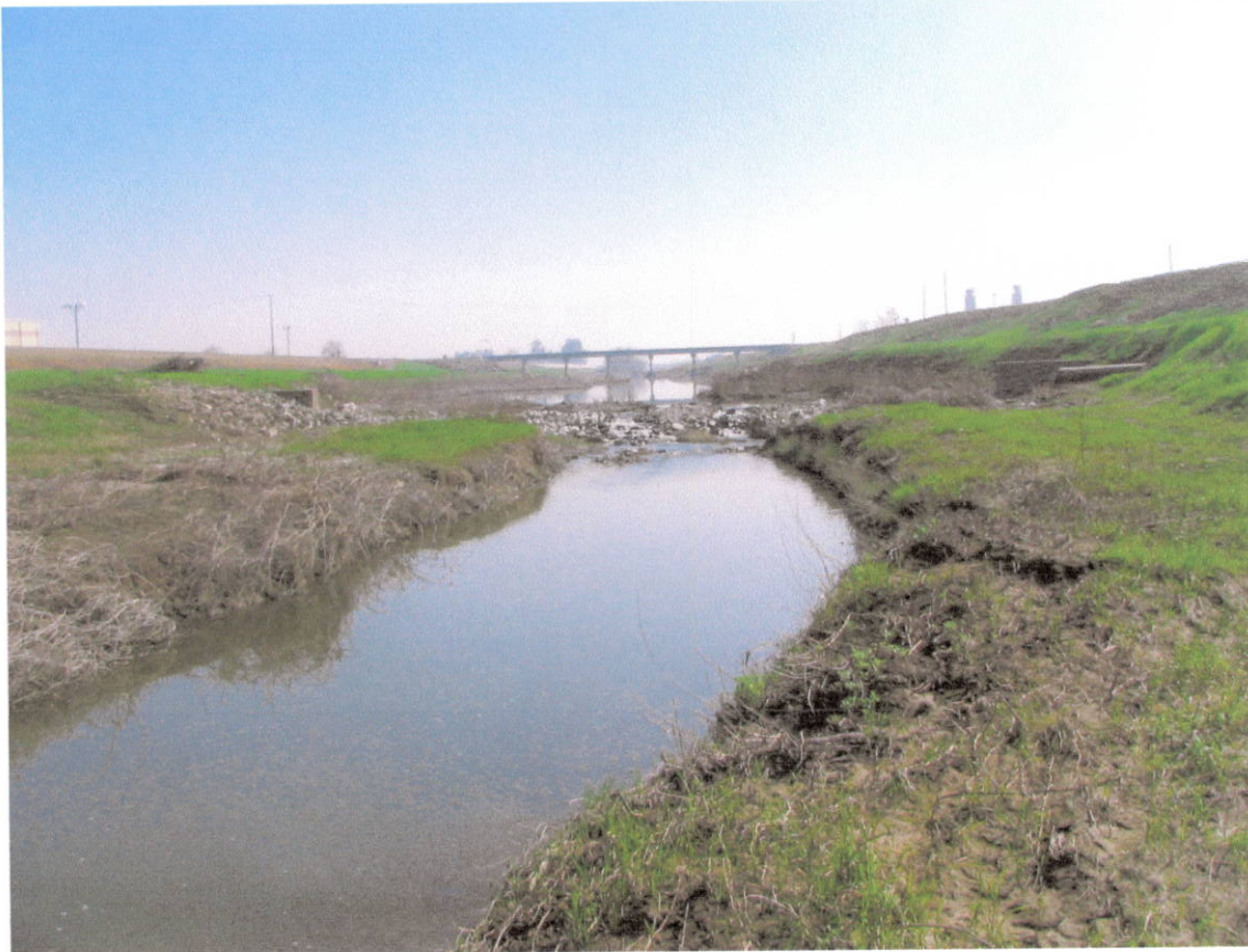
Figure 4. Photo of Budiselich Flashboard Dam, looking upstream with the flashboards not installed.
