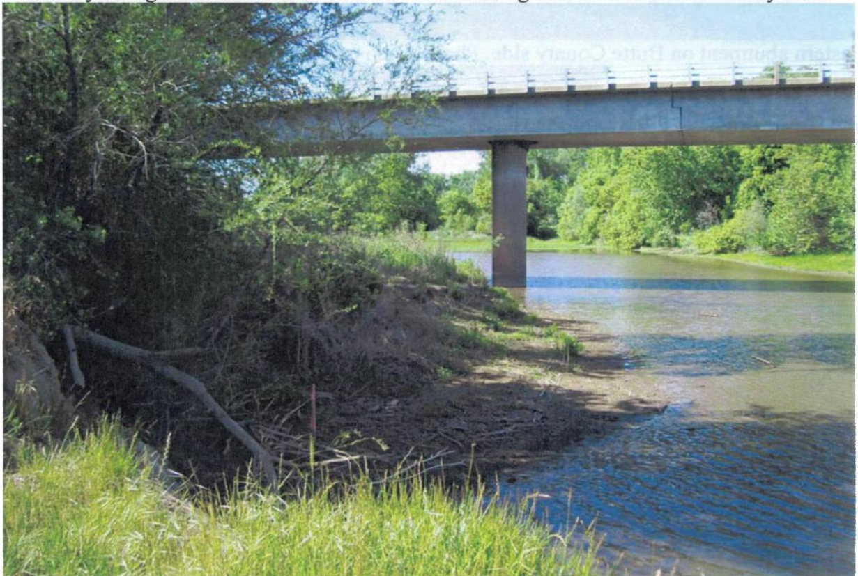
Pier #2 near western abutment. Photo taken looking north toward Glenn County boat launch.
