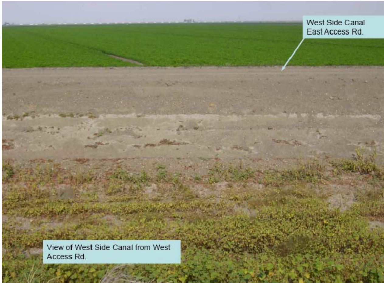
View from Bottom of Kern River Flood Channel to the NE Bank
