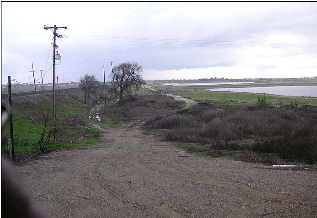
Source: Photograph taken by Reclamation District No. 17 in 2009 Image B: Reach VIID—Looking East
