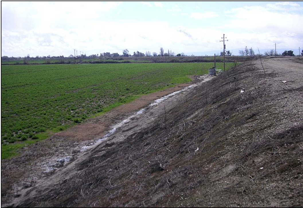
Source: Photograph taken by Reclamation District No. 17 in 2009 Image A: Reach Ic—Looking Upstream
