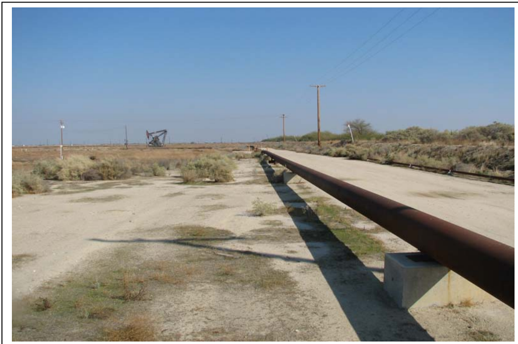
Photo 5B: Picture of Focus Area 3 (Pipeline segment that parallels the Kern River) taken on 11/2/2010, facing north-northeast.
