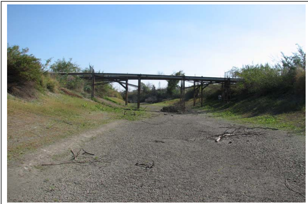
Photo 3B: Picture of Focus Area 1 (Outlet Canal) taken on 11/1/2010, facing south. A pipe bridge supports the section of existing pipelines that cross the Outlet Canal.
