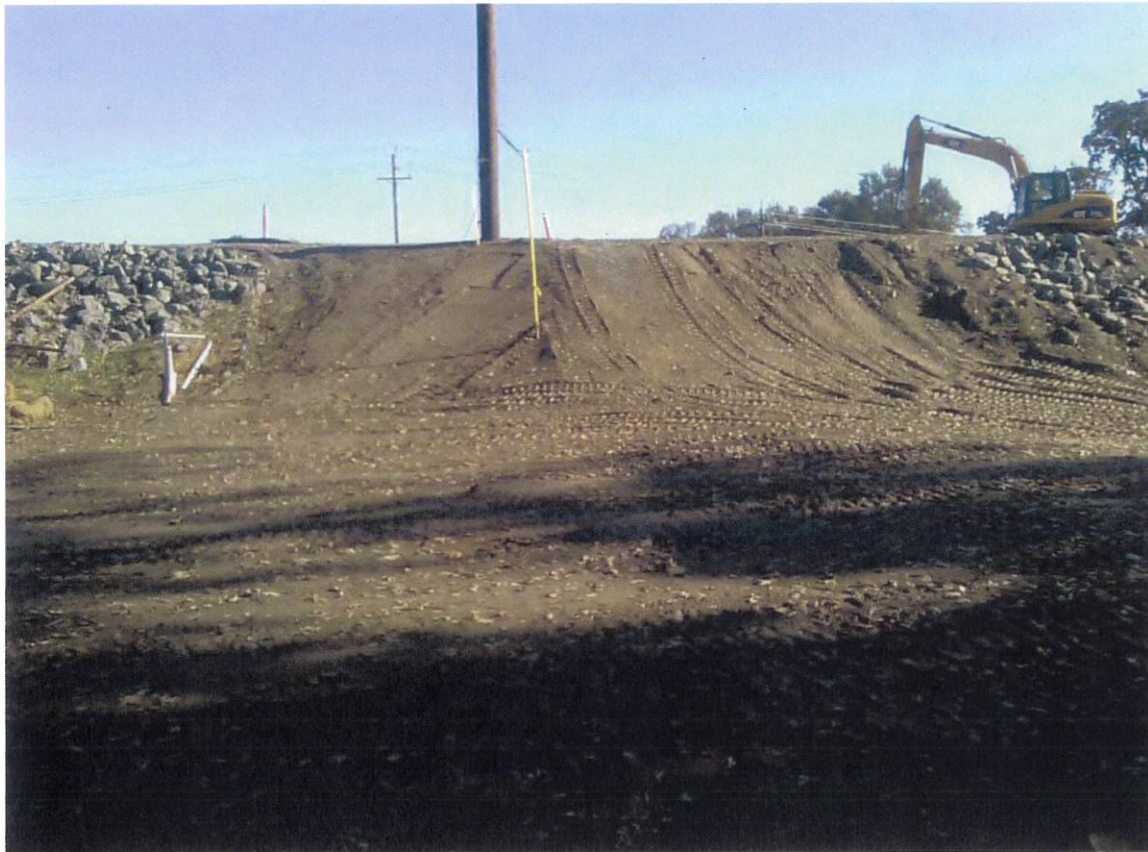
Photograph 3. Looking east from Cummings Pumping Plant on Sacramento River towards electrical service pole at Garden Highway.
