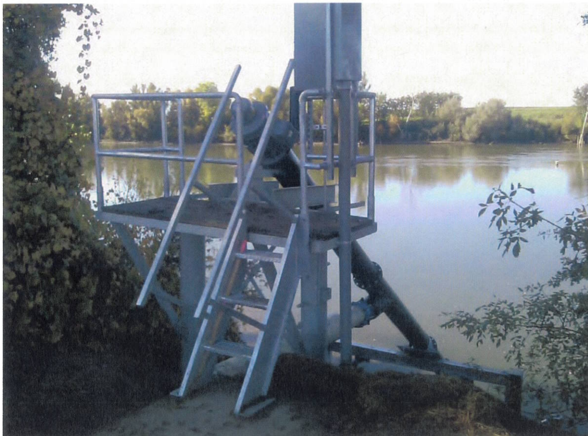
Photograph 4. Cummings River Pump.
