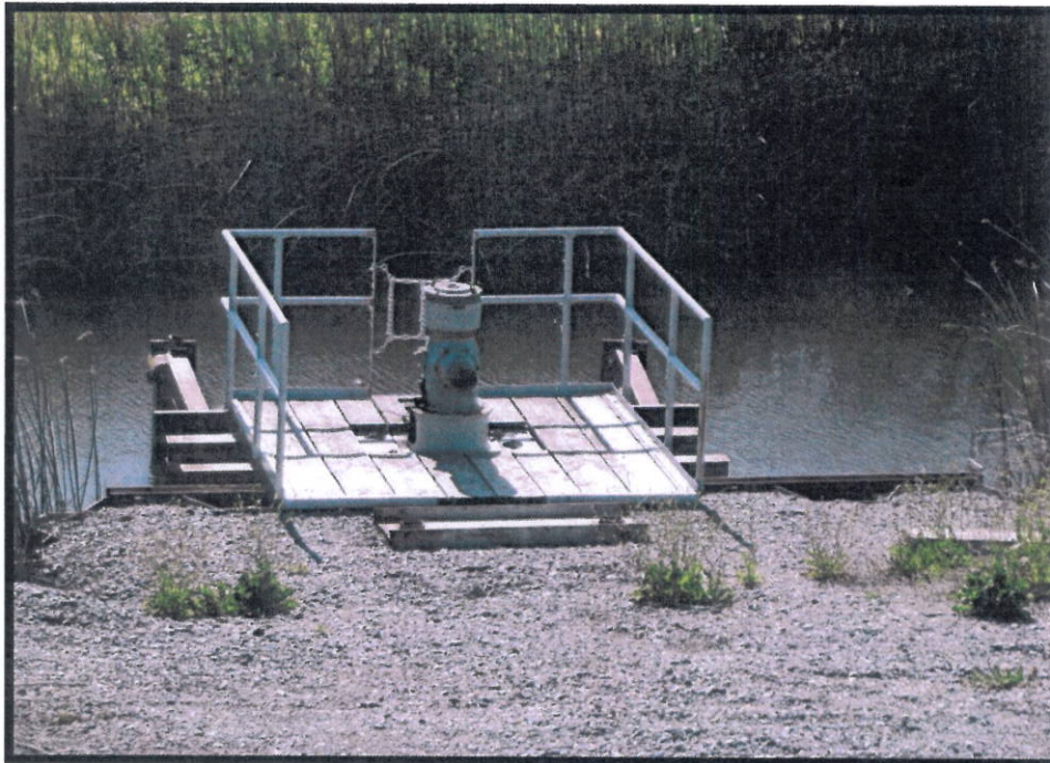
Facing west, landside levee toe, view of sheetpile wall and pump station #12.
