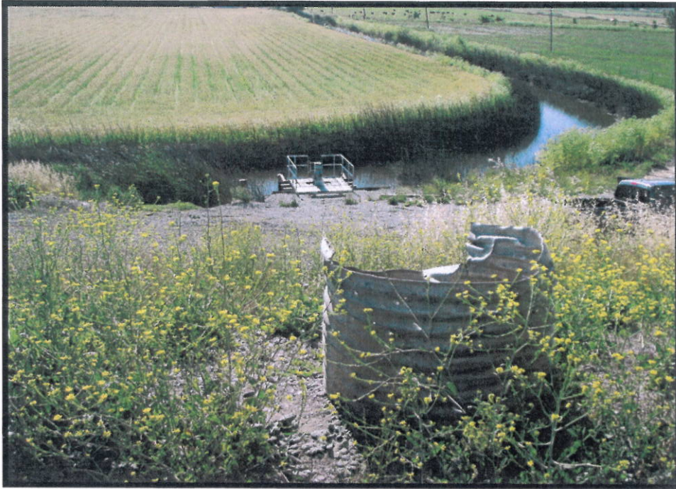
Facing west, landside slope, view of stand pipe on crown and pump at toe of levee.
