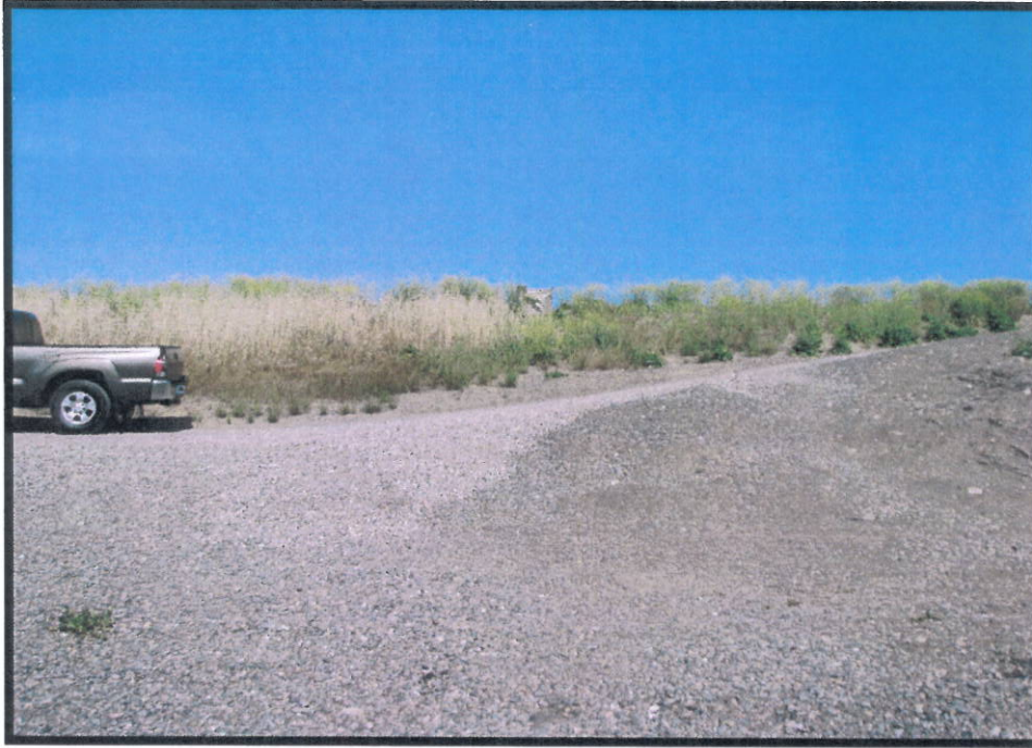
Facing east, landside slope, view of area scoured out by pipe failure, winter 2010.
